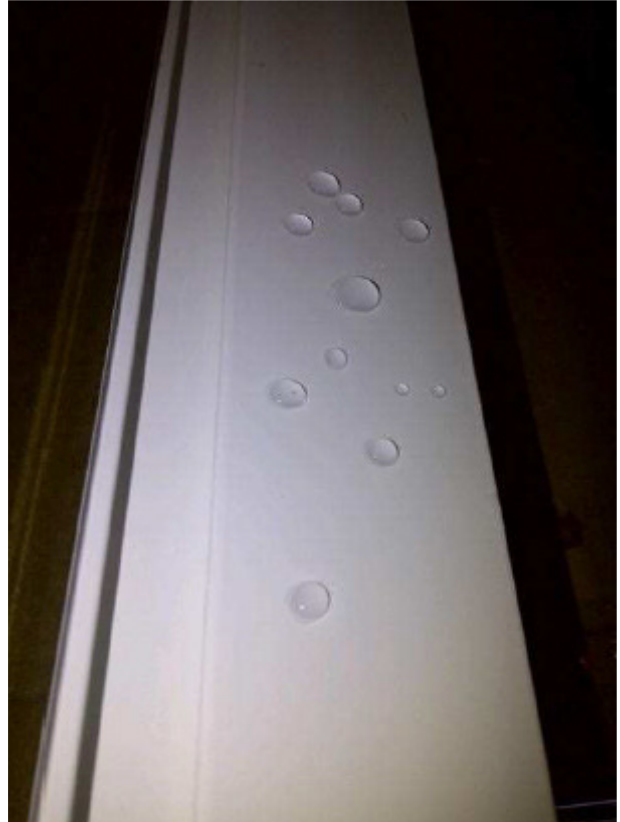
Water Test Photo #2 – Prep Fail
