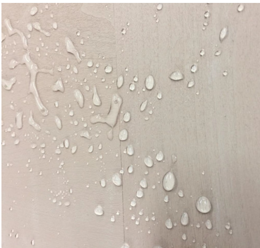
Water Test – FAIL
